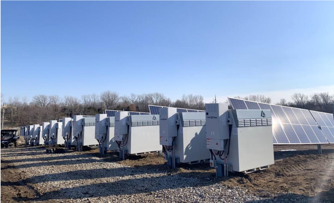
A NEXTracker NX Flow™ integrated solar-plus-storage system. Image: Courtesy of Ideal Energy
